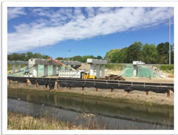
Pier 12; B-602 and B-603 Split Parallel to Tidal Channel
