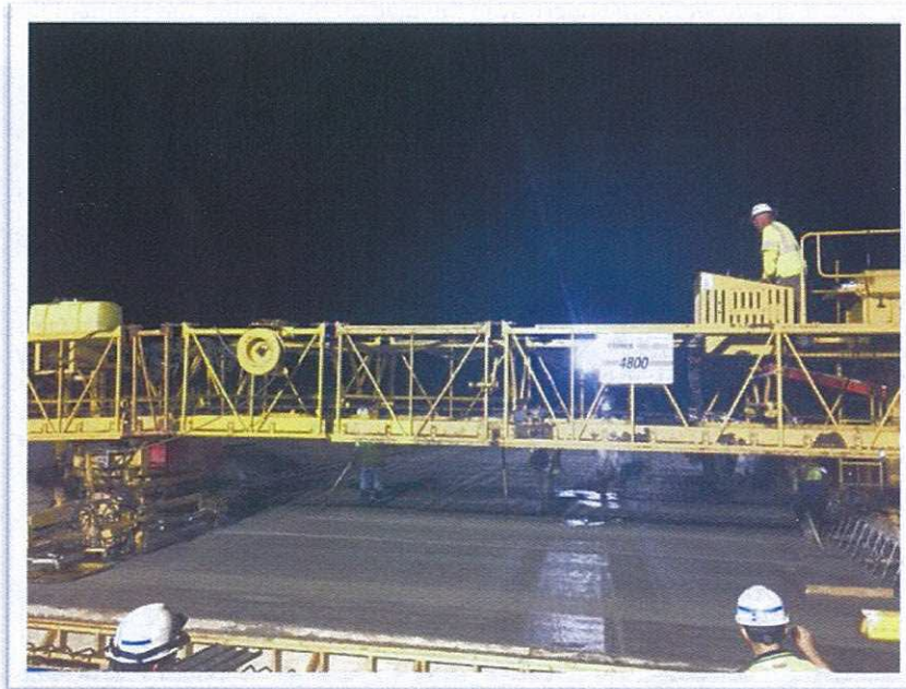
Placement of Deck Concrete for the I-64 Westbound Bridge over Industrial Park Drive
