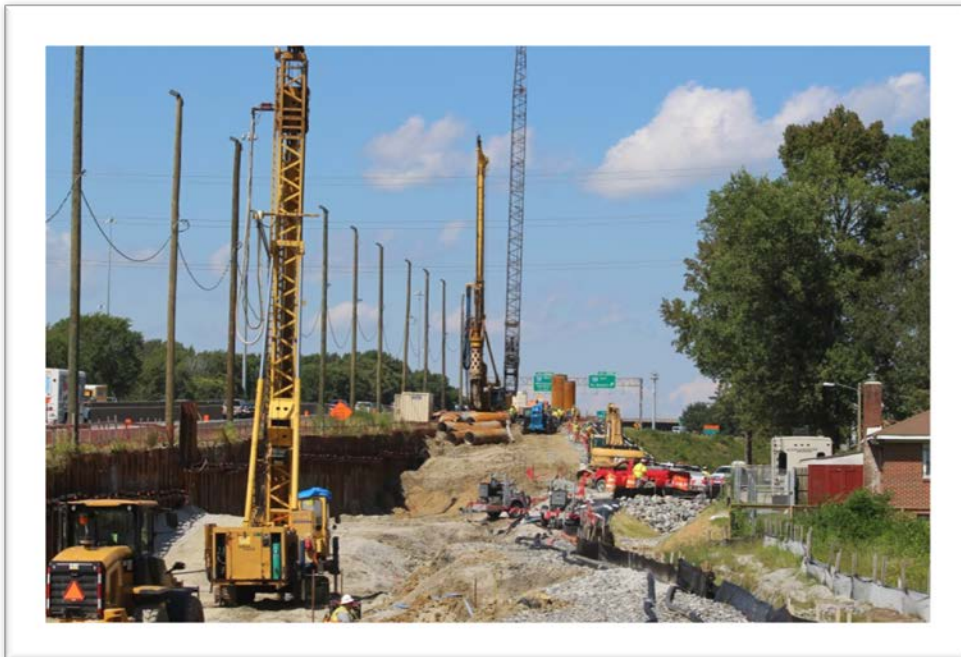
Densified Aggregate Pier Drilling (foreground) at Retaining Wall M and P (I-64W)
